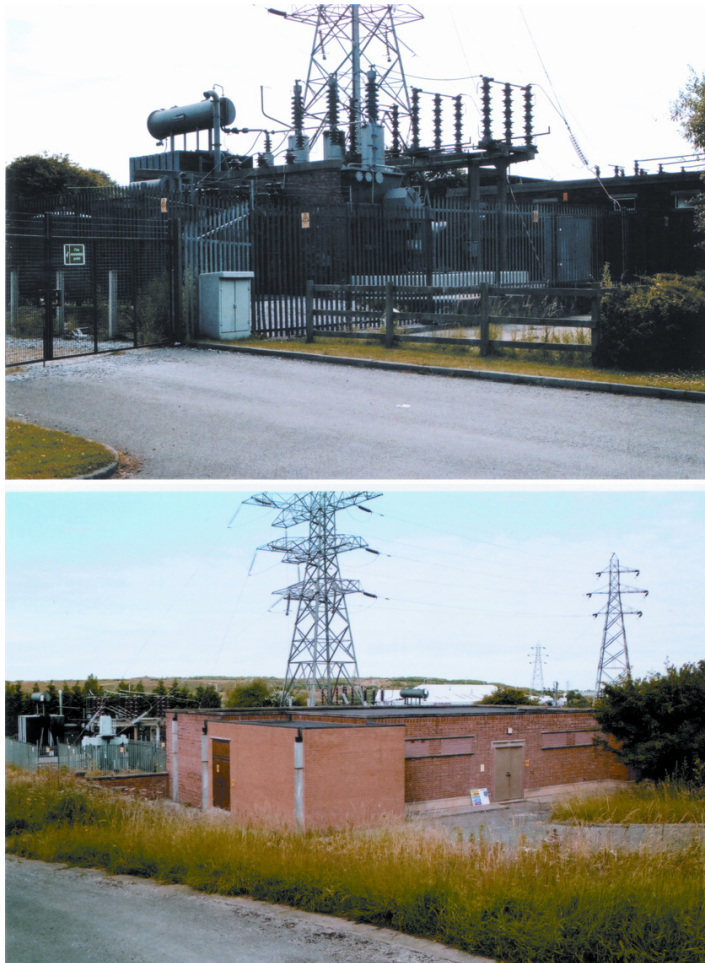
Figure 8.6: An existing electrical substation (Wallasey)
